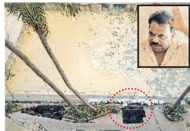
The sinkhole (circled) in which watchmen Raman Mangela (inset) and Mahendra Ram fell
